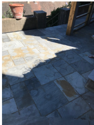
Photo showing five spot method showing through to the surface and the discolouration after an Acid cleaner has been used and left to dwell. Please do not use either of these methods.
